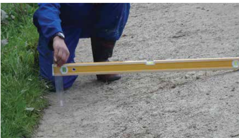
The camber on this track is too steep.
