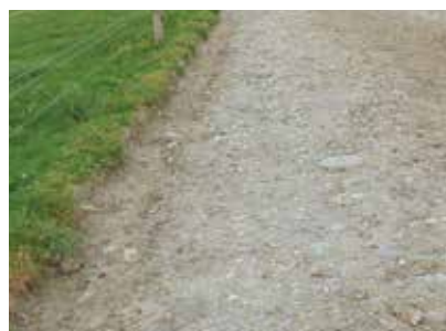
Bad surface layer
