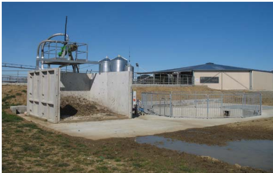
Solid separator with bunker and effluent storage tank
