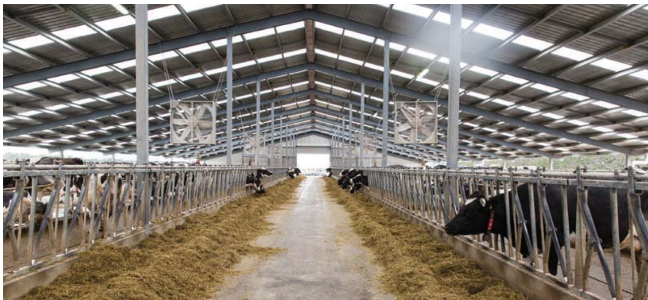
Low speed fans above feeding passageway
