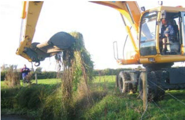
Fence positioning which allows a long digger to reach over the top.
